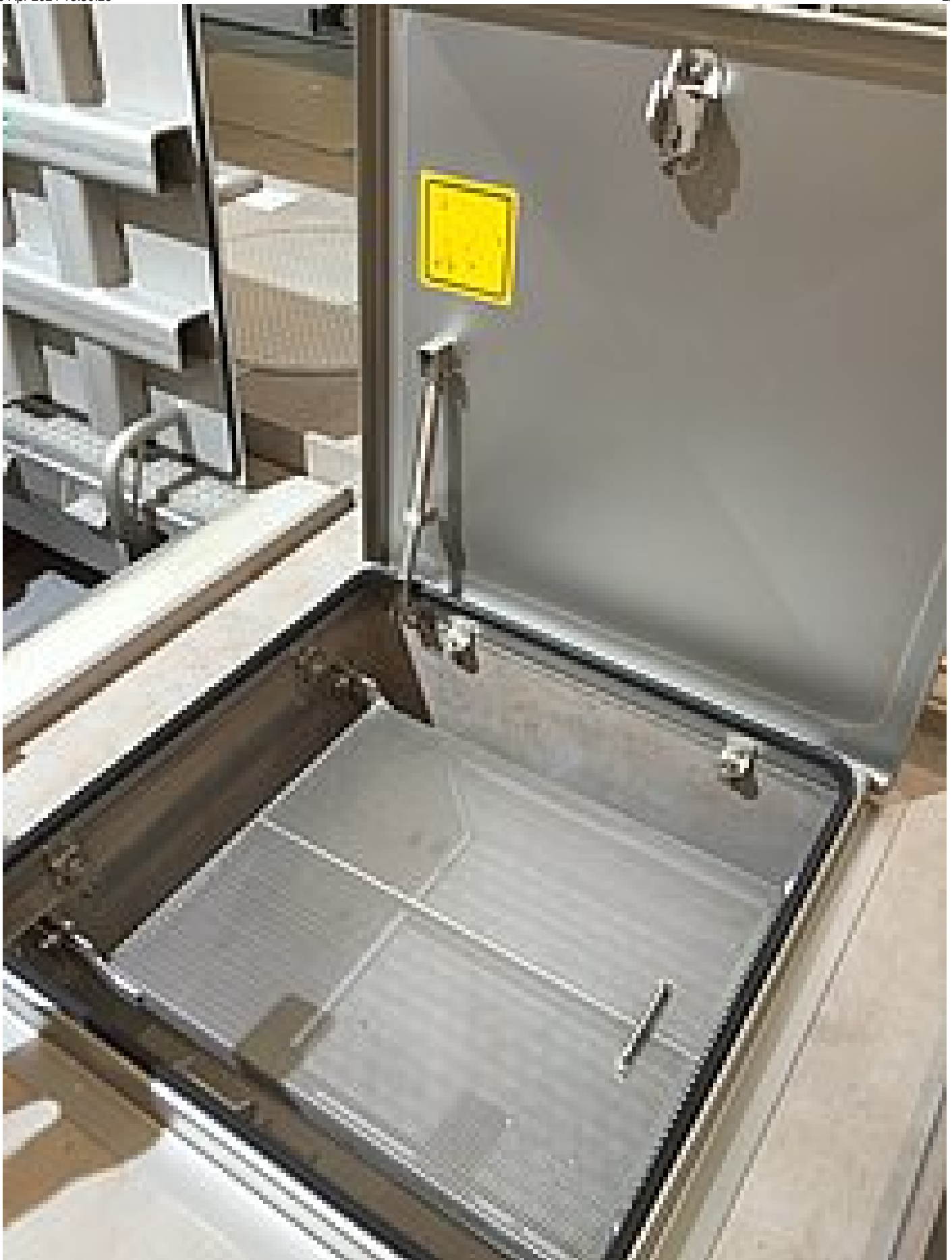
Manhole cover with antifall guard – closed
