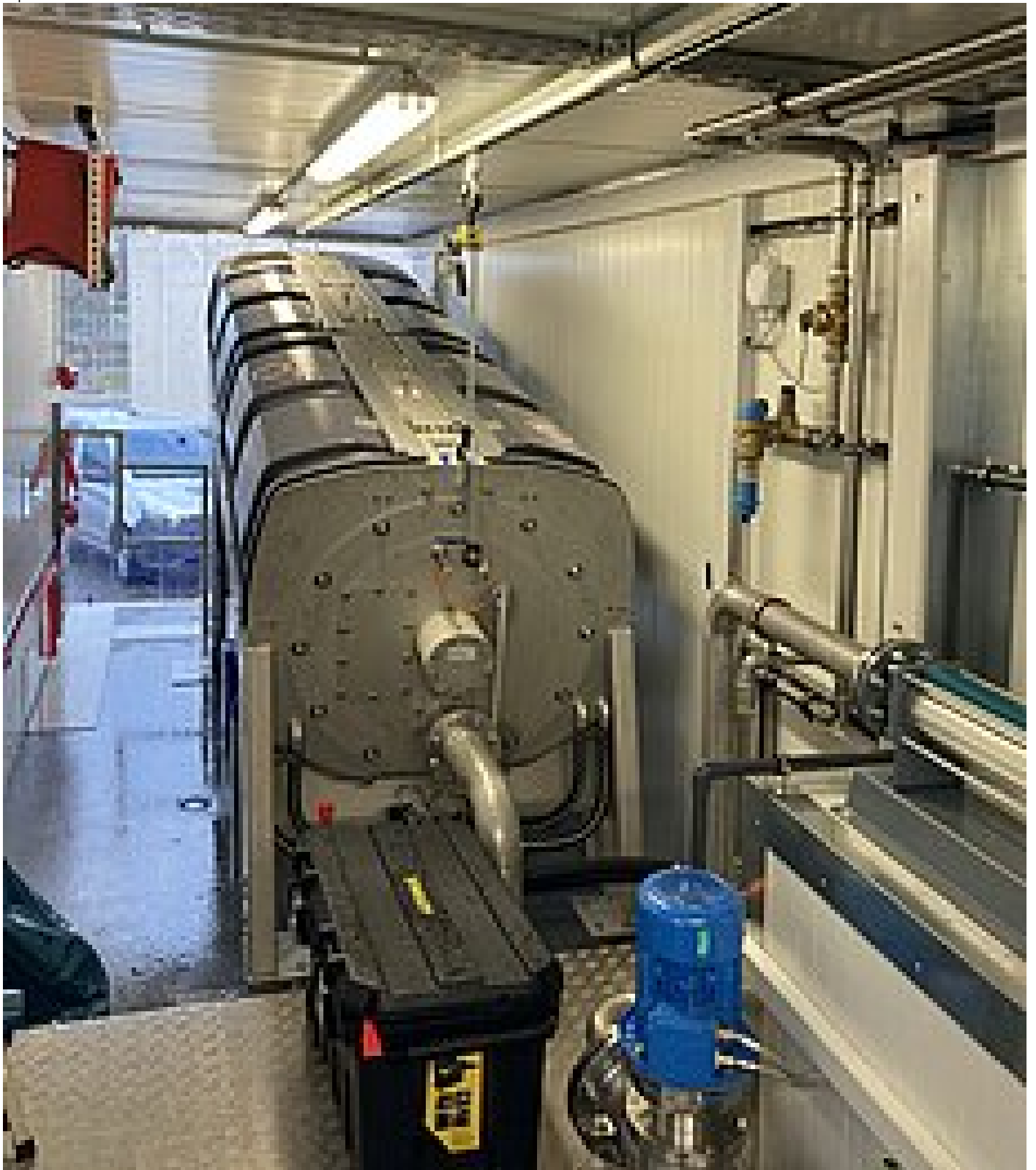
HUBER Screw Press Q-PRESS®, installed in a semi-trailer
