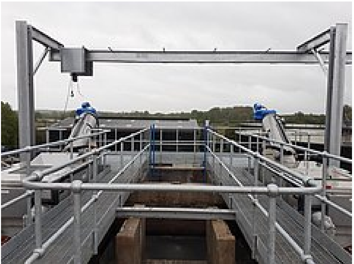
2x HUBER Sludge Acceptance Plant ROTAMAT@ Ro3/1200/355 units installed at Wanlip STW
