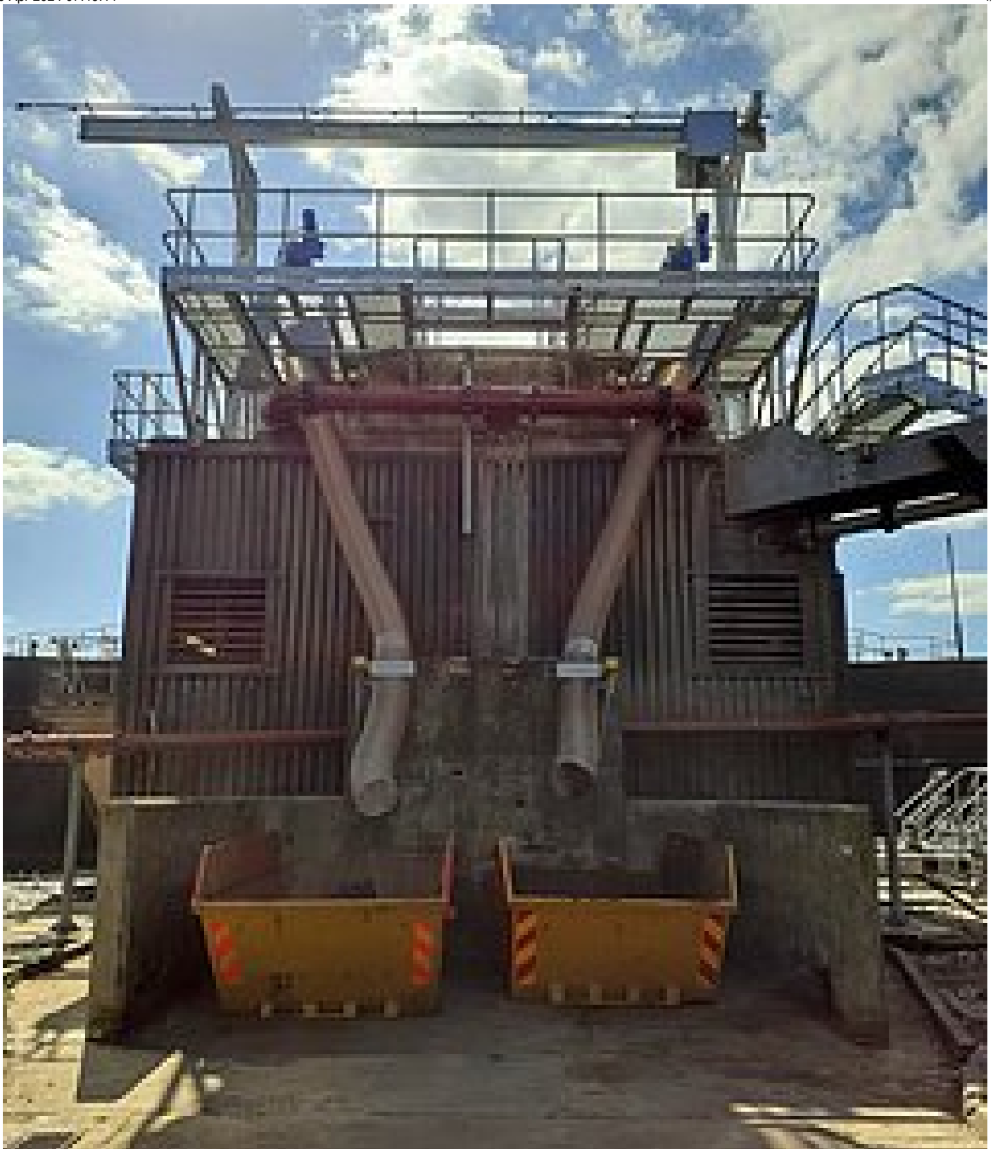
New screens and discharge chutes
