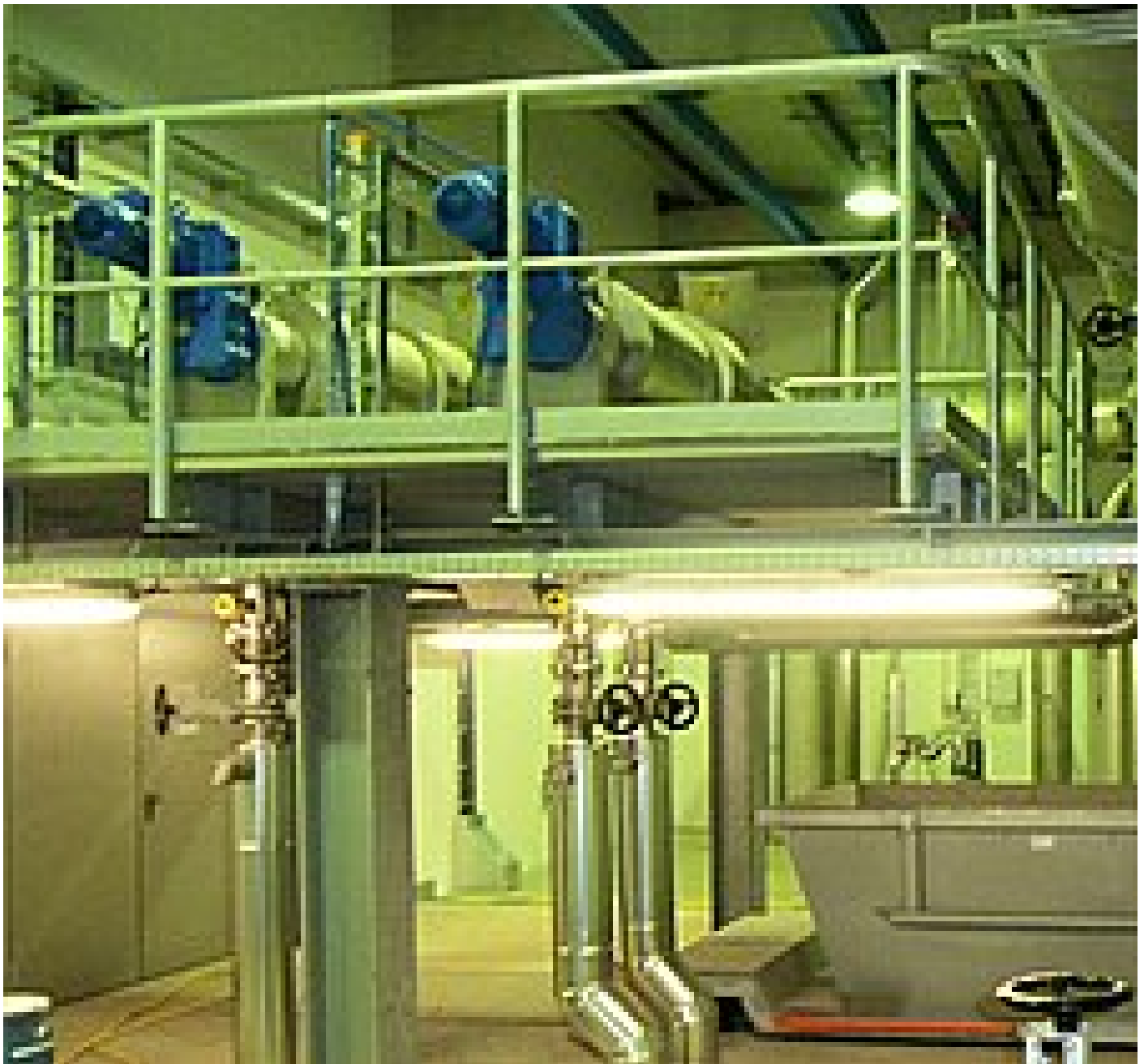
Two insulated STRAINPRESS® machines for grease sludge screening, below a container into which the screenings are discharged
