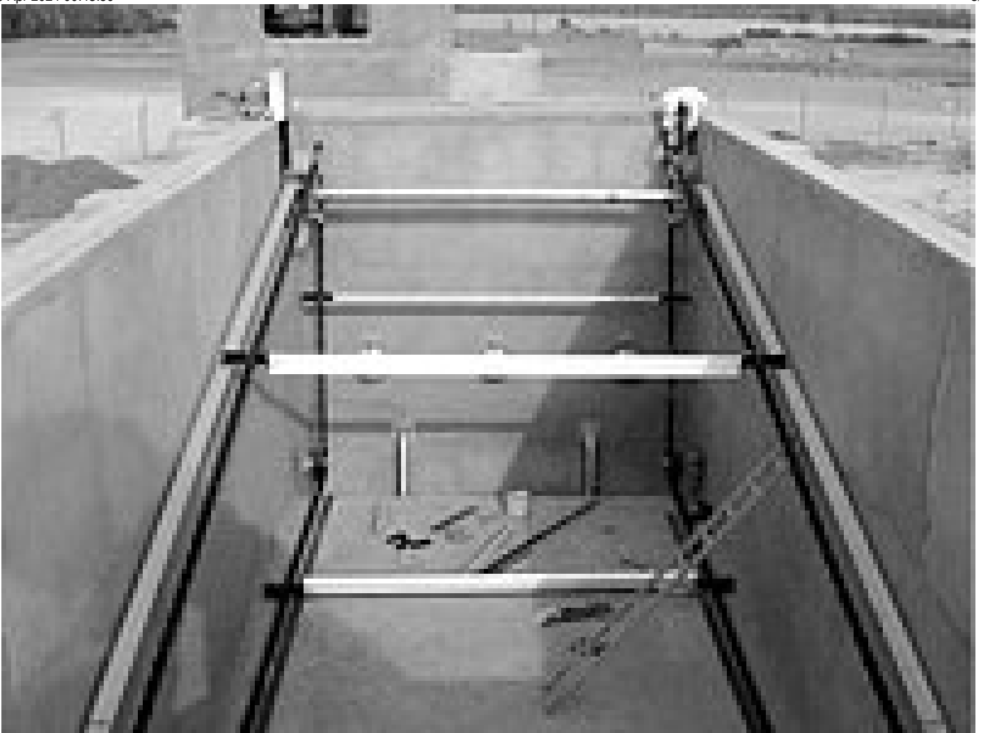
Sedimentation tank before start-up
