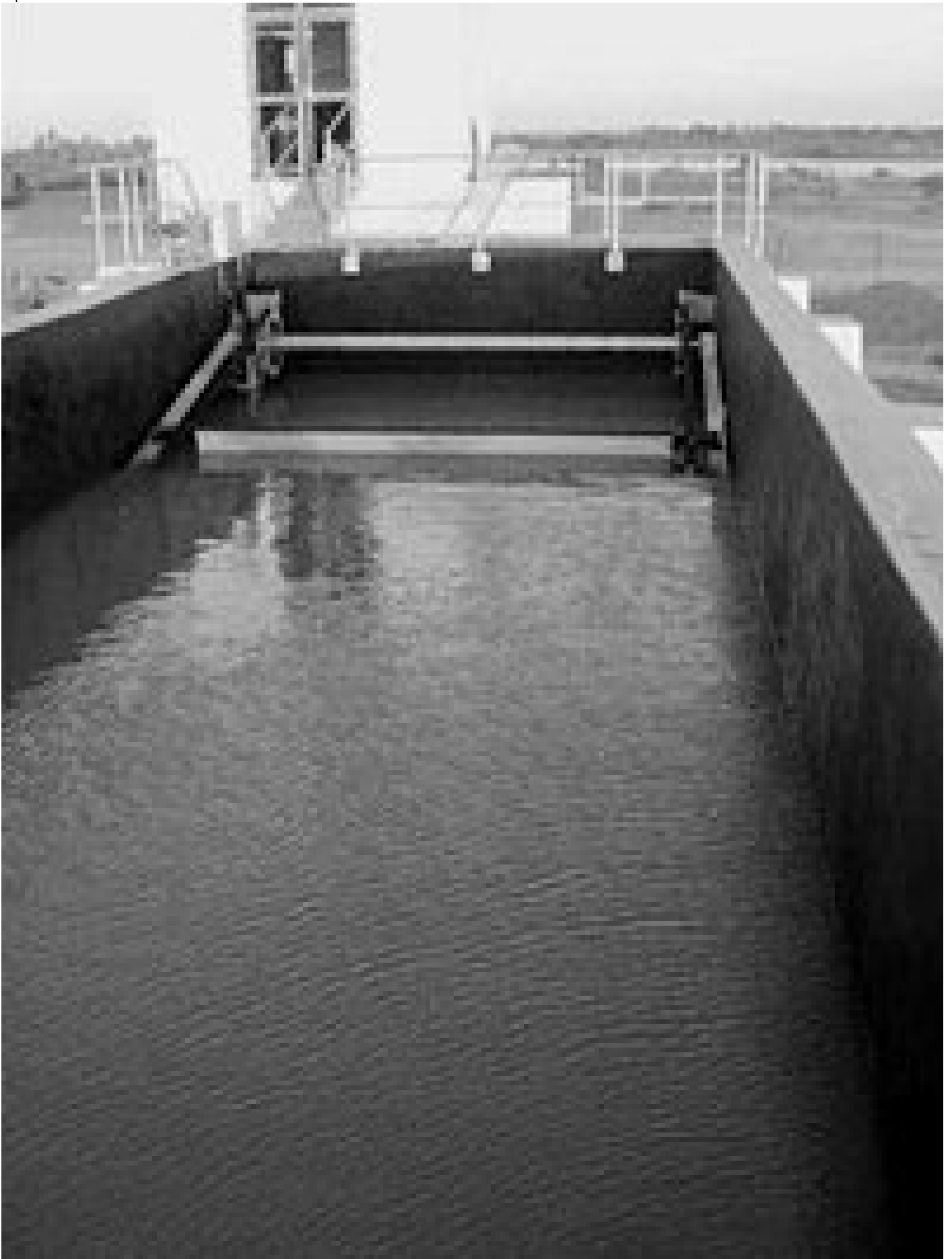
Filled sedimentation tank
