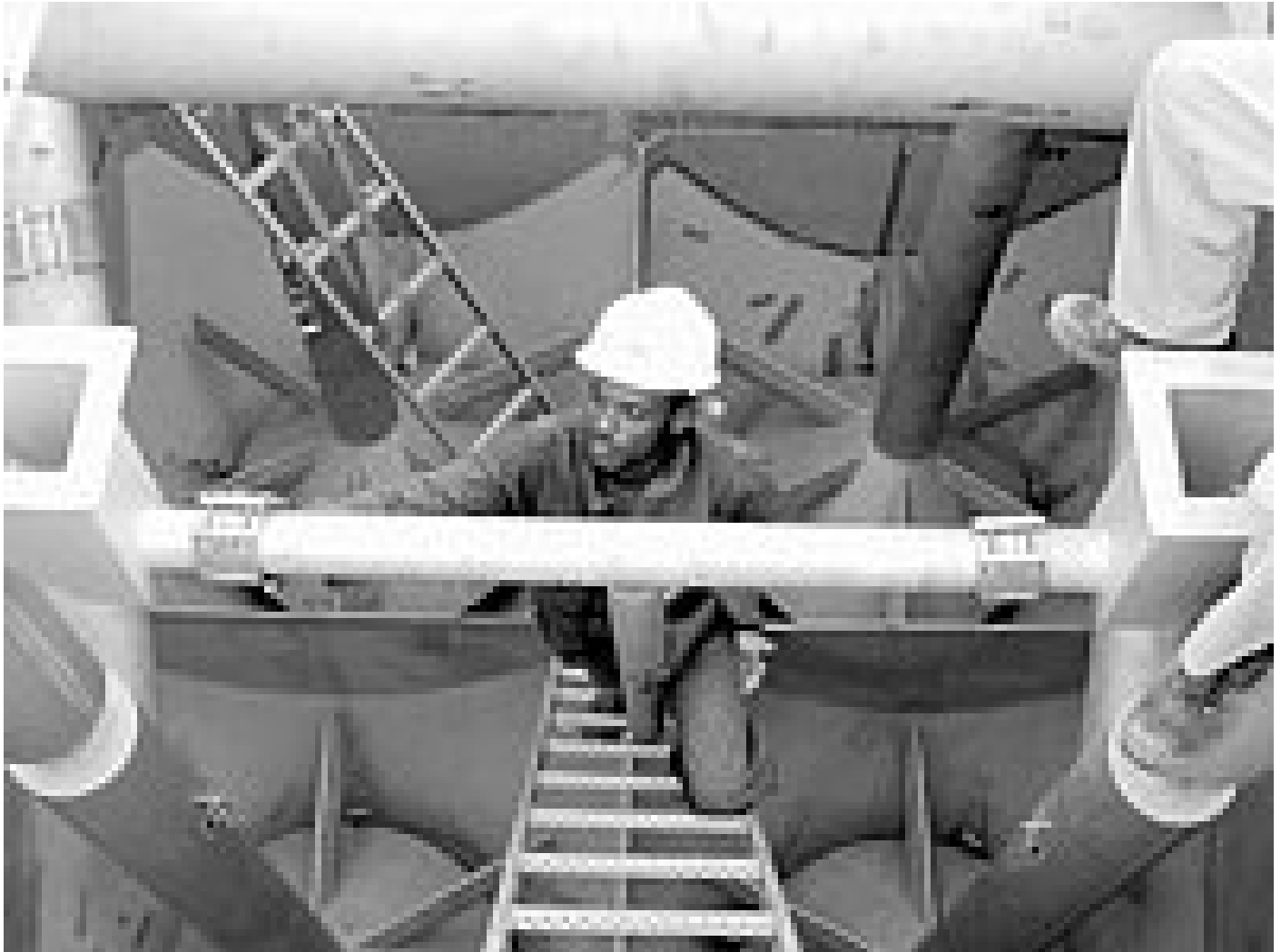
Interior of a Sandfilter
