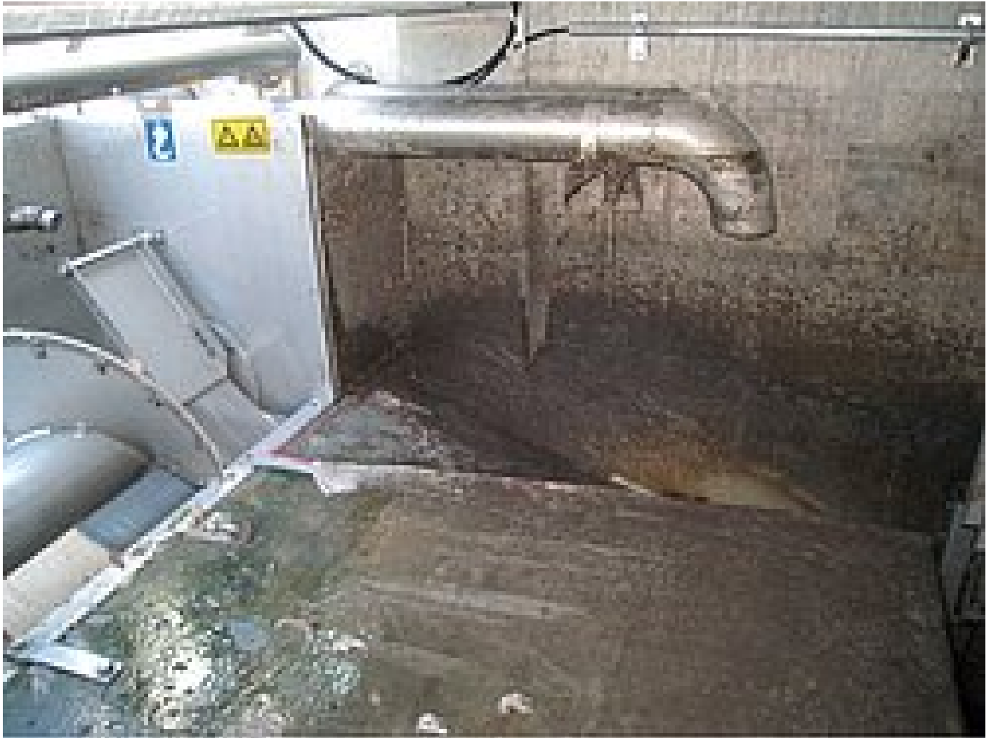
Screening launder channel built into the berm, washing system at the left, discharge line on top
