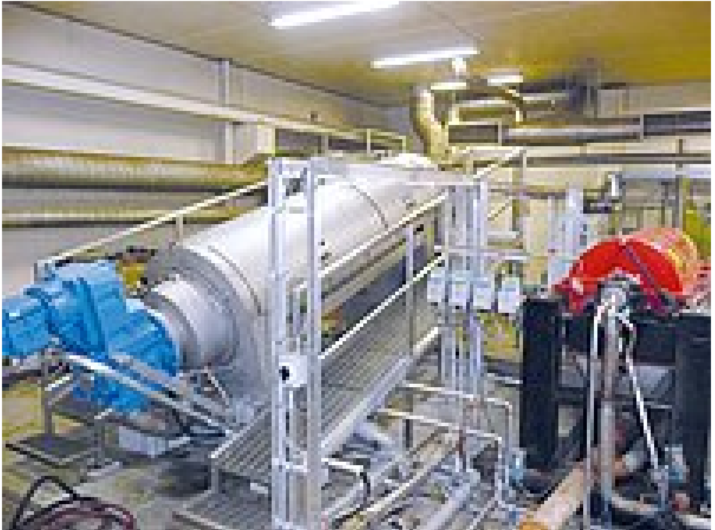
Screw Press RoS 3Q 620 beside the maintenance-prone decanter
