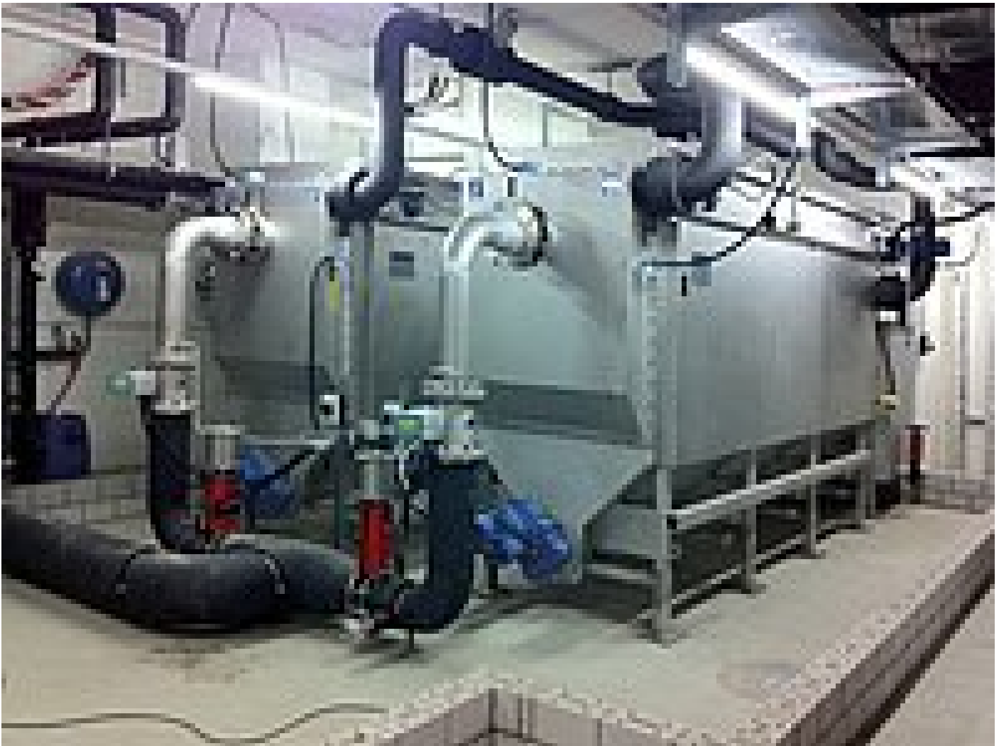
Two RoWin Heat Exchanger size 8 installed in the second basement of the Wintower building at Winterthur
