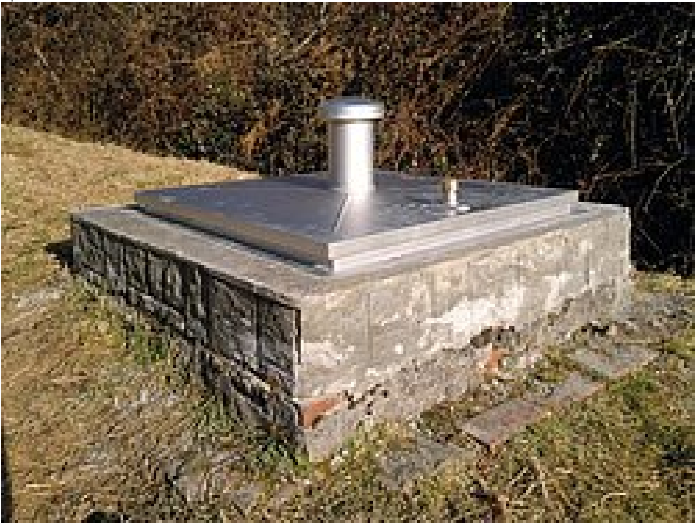
Weatherproof manhole cover
