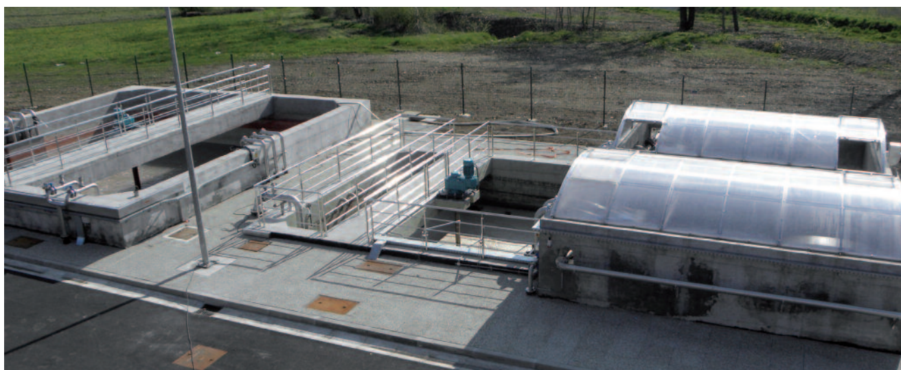
Mixing and balancing tank, bio-tank and HUBER MBR system
