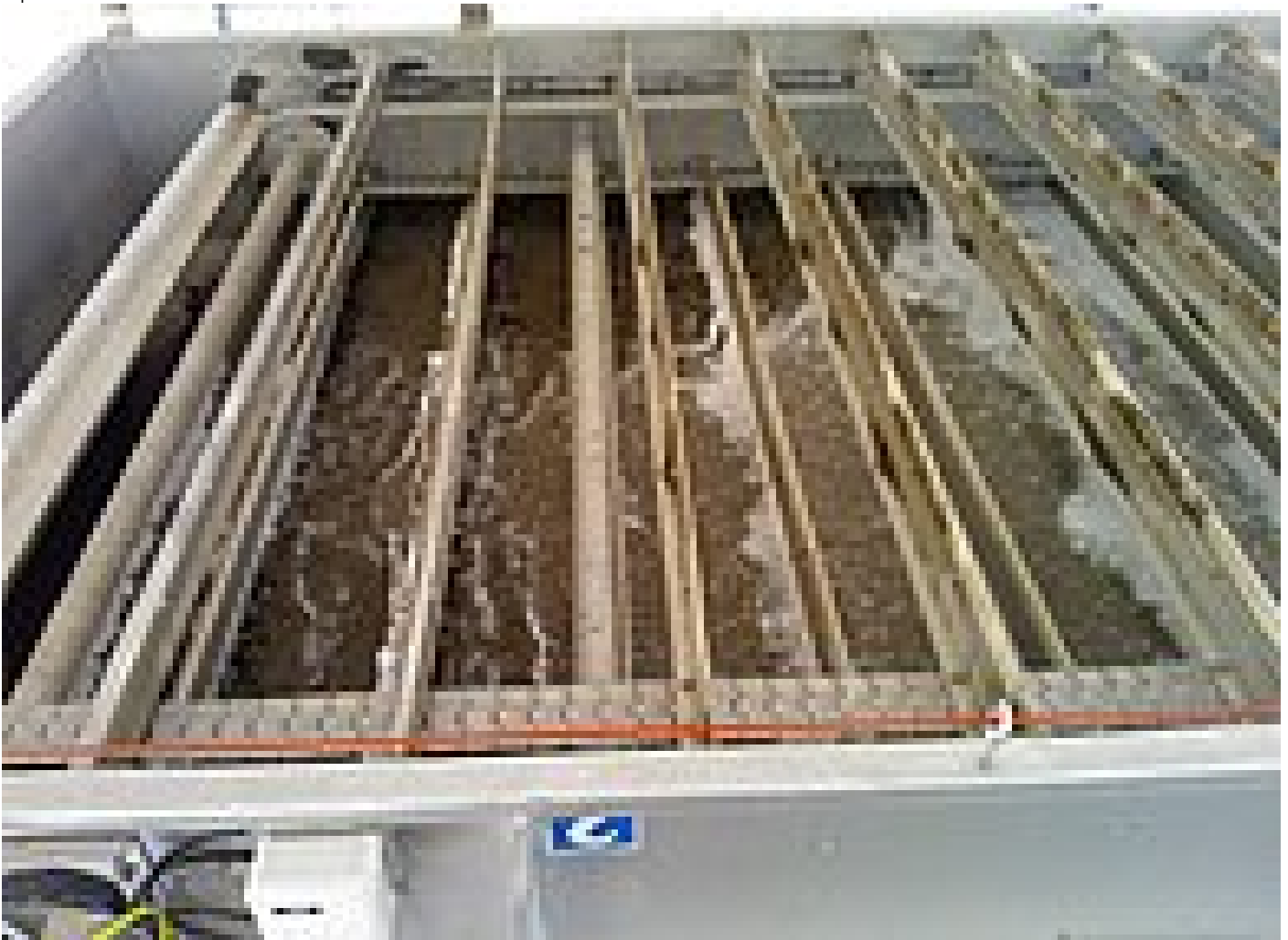
View into the HUBER Dissolved Air Flotation Plant HDF
