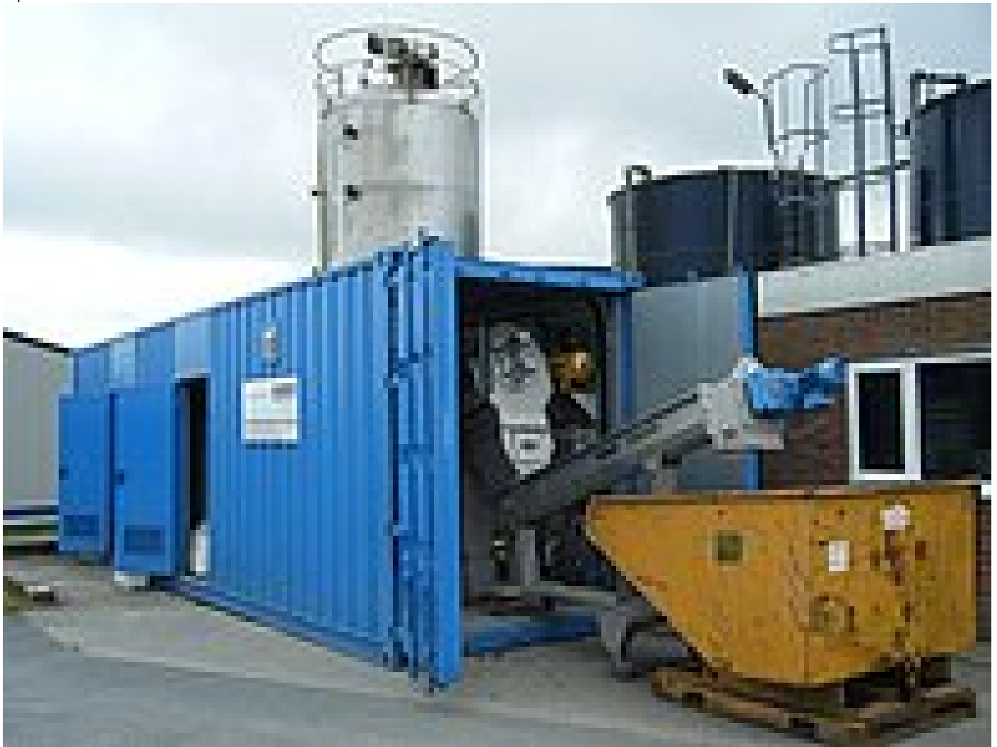
Trial plant on test at Dairy Crest
