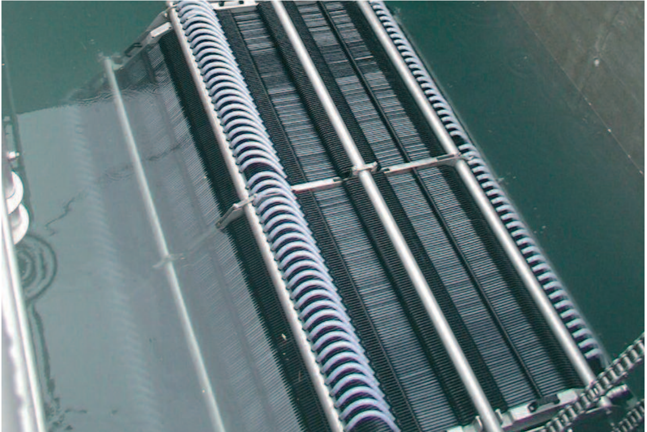
Membrane filtration chamber prior to start-up
