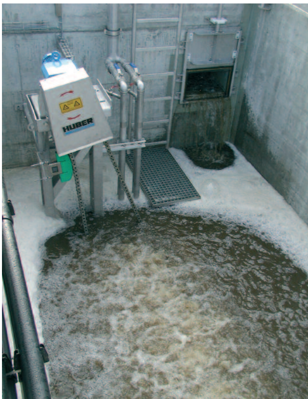
VRM® Membrane Filtration Plant
