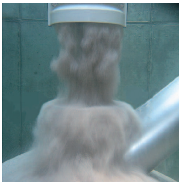
Crystal-clear effluent from the sandfilter
