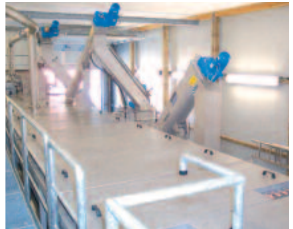
Complete Plant Ro 5 discharging the screenings into a Super Launder Washpress WAP/SL
