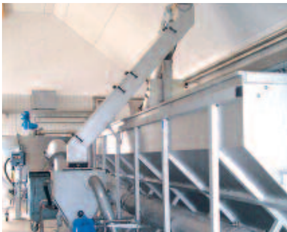
Indoor removal of screenings, grit and grease without odor nuisance
