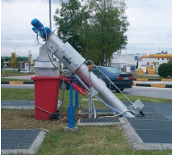
ROTAMAT® Micro Strainer installed in the center of a traffic circle
