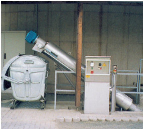
Outdoor installation with electrical heating and thermal insulation for frost-protection
