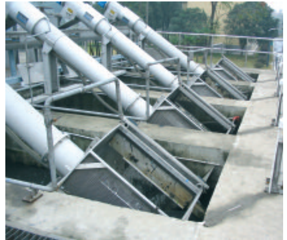
Four ROAMAT® Fine Screens Ro 1 installed in parallel channels
