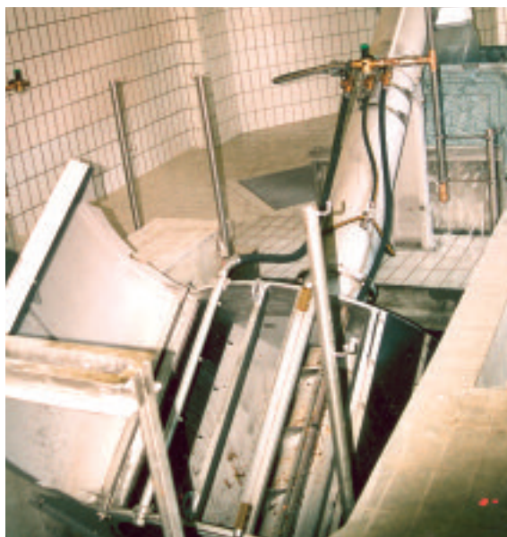
ROTAMAT® Fine Screen Ro 1 installed in a channel; with integrated screenings washing (IRGA) and spray guard
