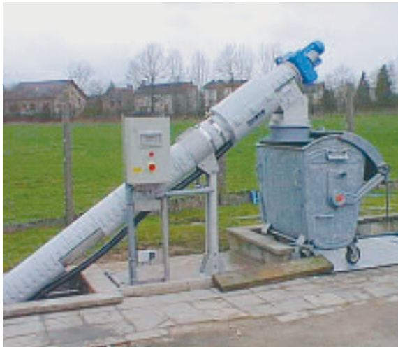
Outdoor Installation with frost-protection and bagger
